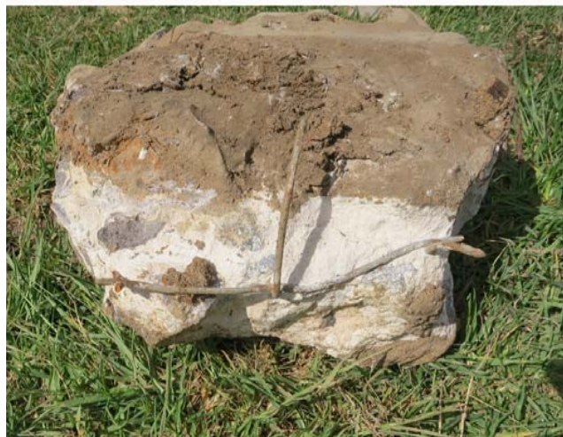
Piece of the old roadway showing original reinforcing
