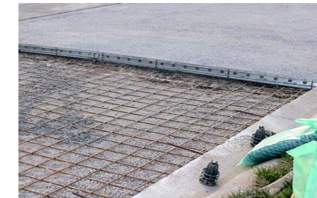
End of day's work showing expansion joint and mesh ready for the next day's pour
