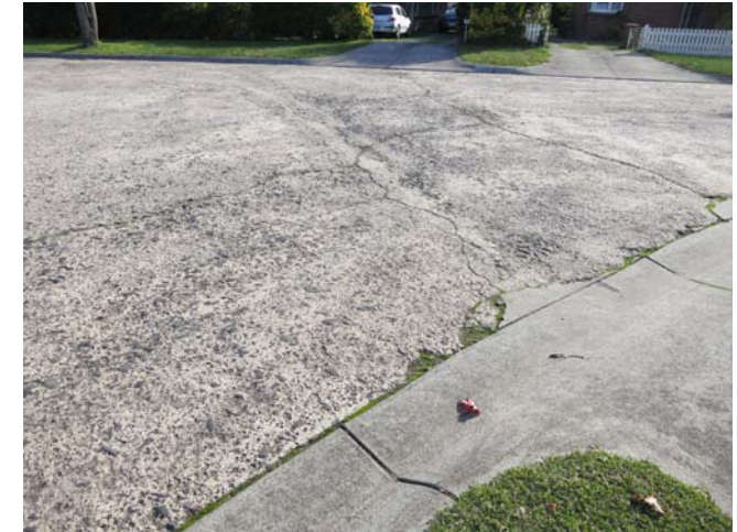
This 2014 photo of the corner of Sherwood and Woodstock Roads shows the concrete roadway today. Note the extensive cracks, the large aggregate embedded in the cement, the replacement low profile curbing installed in 1991 and one of the original shallow surface drains running from right to top left.
