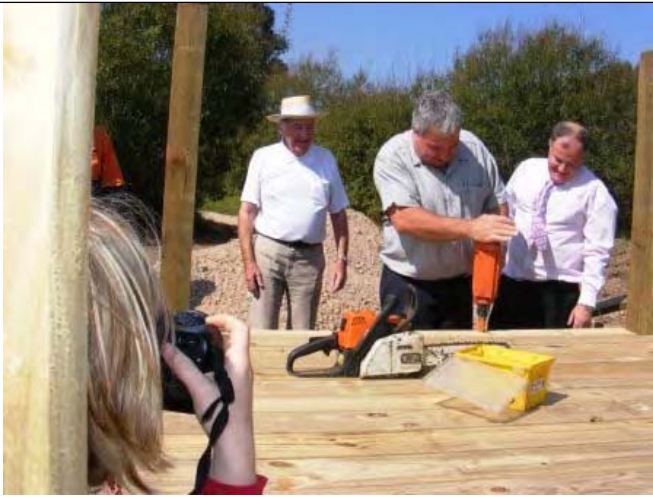
Leo demonstrating his carpentry skills in laying the last plank of the four board walks
