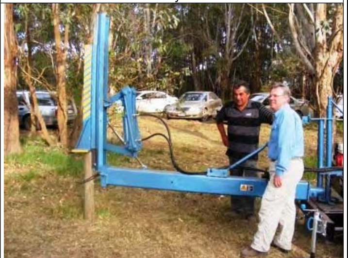
Philip won the raffle and had the honour of driving the 1 st pile using Branco's specially built pile driver
