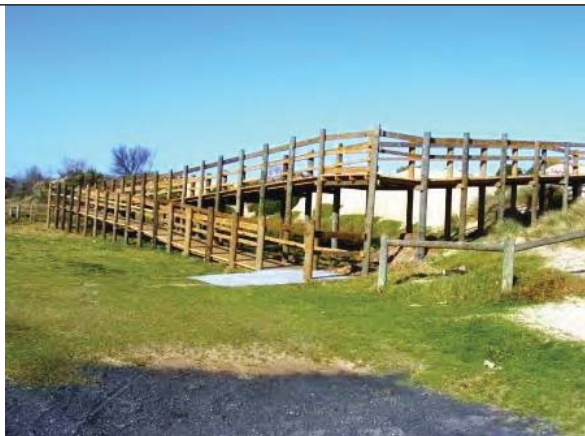
The wheel chair access ramp at Seaspray nearly complete as a consequence of the Club's $10,000 contribution
