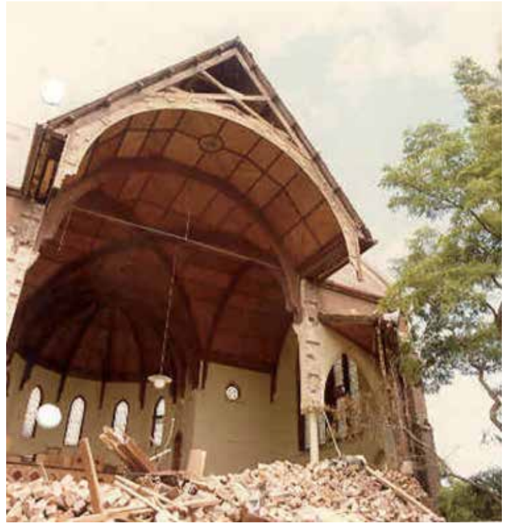
Unauthorised demolition of Wesleyan Methodist Church c1985 to 1986 Stonnington History Collection PH10189.11
