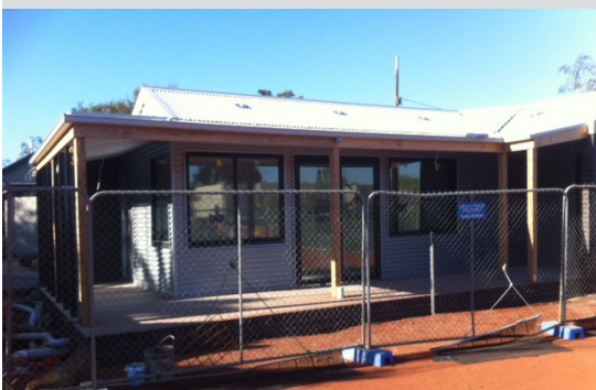
Partly completed new clubhouse for the Glendearg Malvern All Saints Tennis Club 2014 (John Richards)
