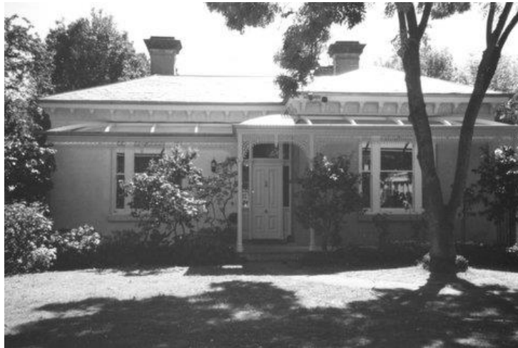
Christian Benjamin and Caroline Finger's house in Weinberg Road (now Wattle Road), Hawthorn being restored, March 2003. Source. G. Dovile.
