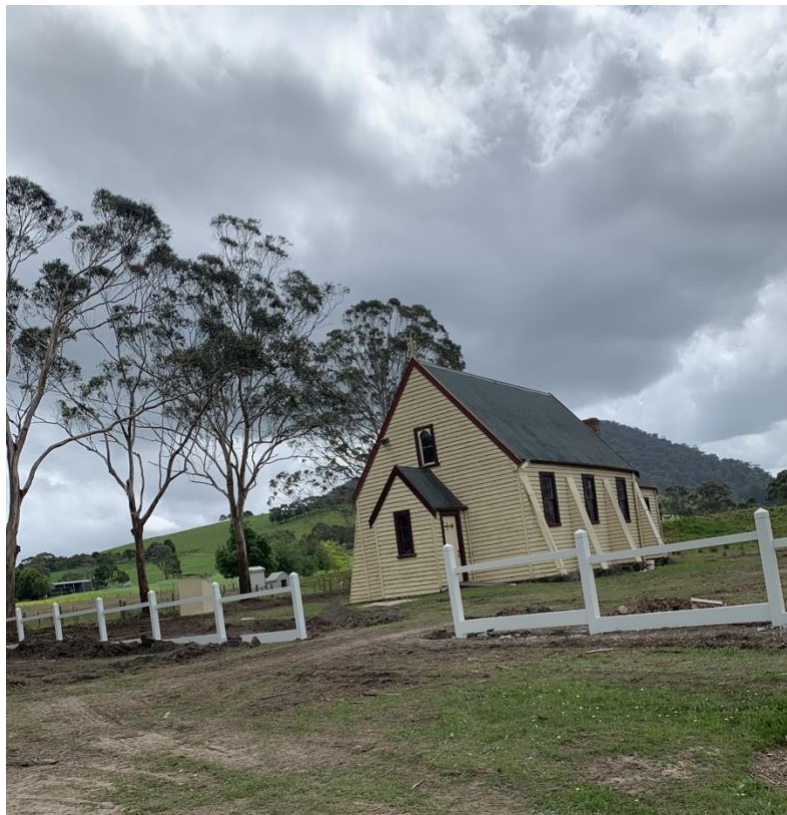
The former Scotsburn Union Church, being restored in October 2023, with trees cut down and new fence being installed.
